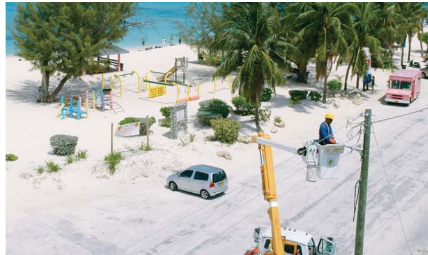
Caribbean Utilities owns and operates approximately 550 kilometres of transmission and distribution lines and 22 kilometres of high-voltage submarine cable.
