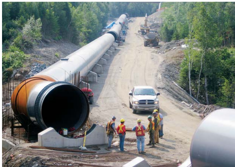
A $17 million refurbishment of the Rattling Brook hydroelectric generating facility, the largest capital project in dollar terms ever undertaken by Newfoundland Power, was completed in 2007.
