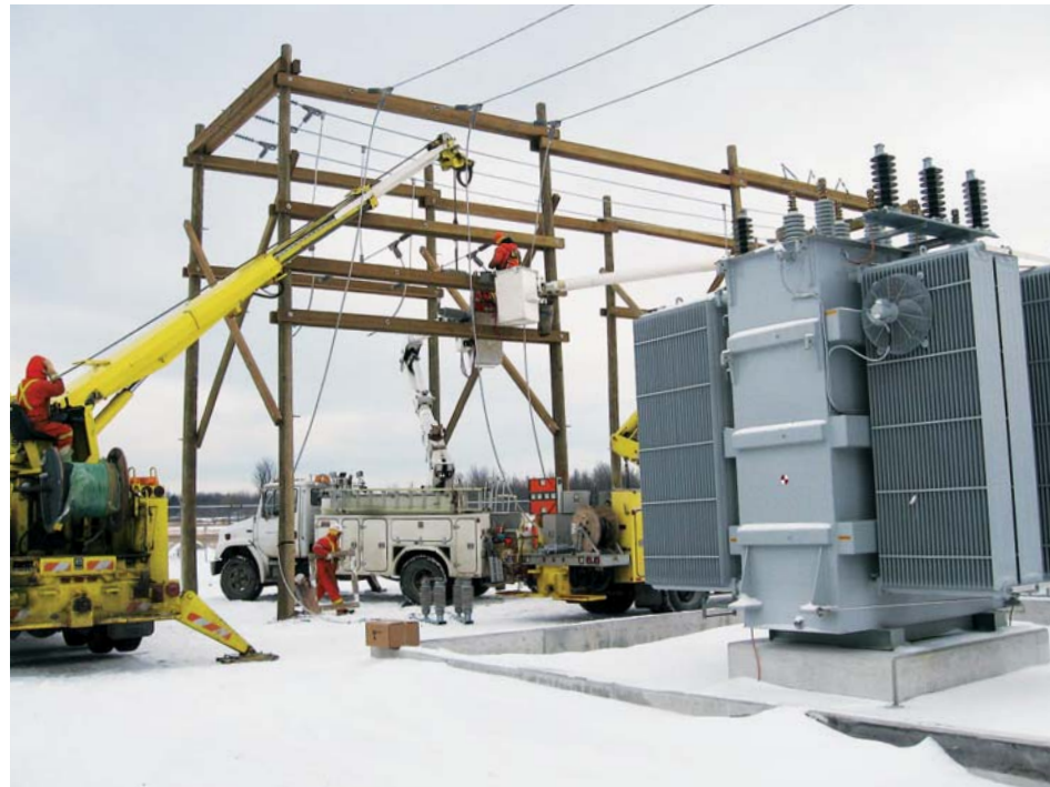
In 2007, a new $1.4 million substation was commissioned in Gananoque, providing improved reliability and security of service to the community.
