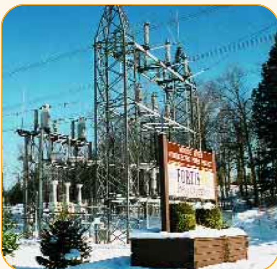
Moose River has a generating capacity of 12.5 MW.
