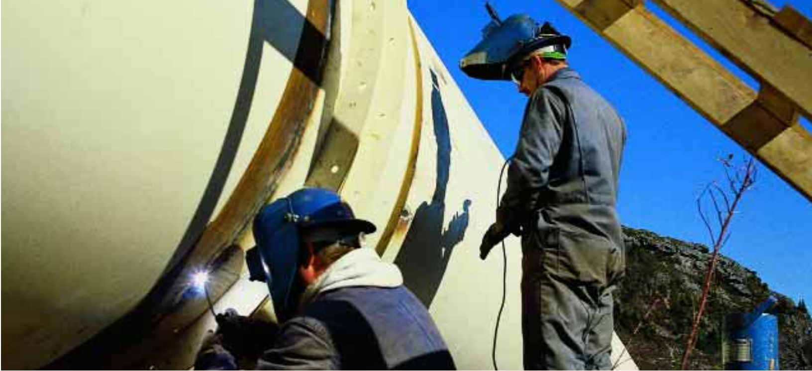
Newfoundland Power invested in upgrades to hydroelectric plants such as replacement of the Horsechops penstock.
