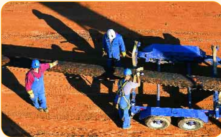
More than 200 kilometres of electricity lines were rebuilt in 2000 to improve reliability of service.
