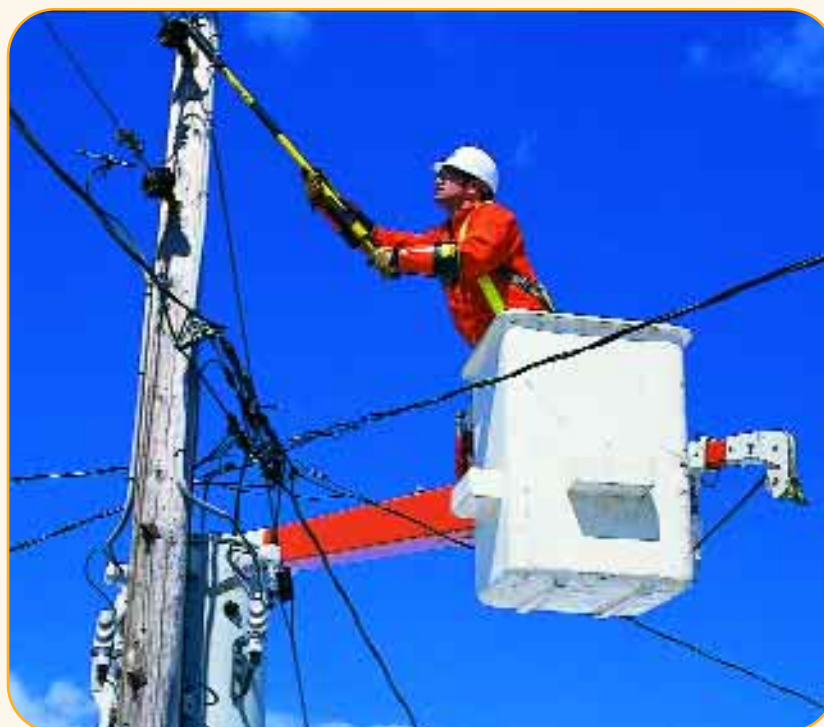
Capital investment programs contribute to system and reliability improvements.
